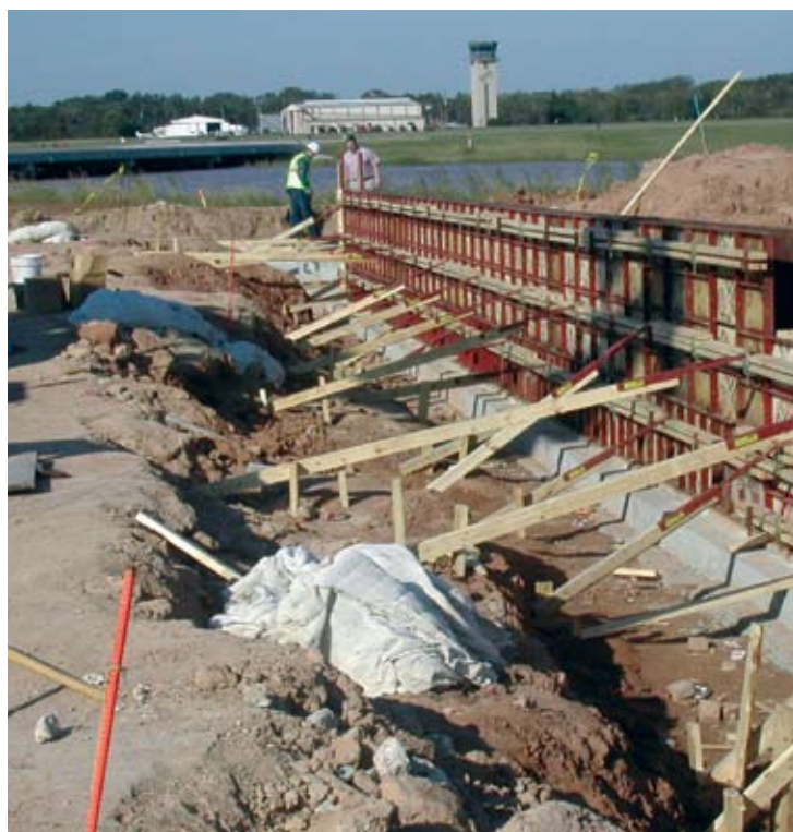
Currently, utility work—water, wastewater, fire protection—is under construction on the 66-acre plot of land.
